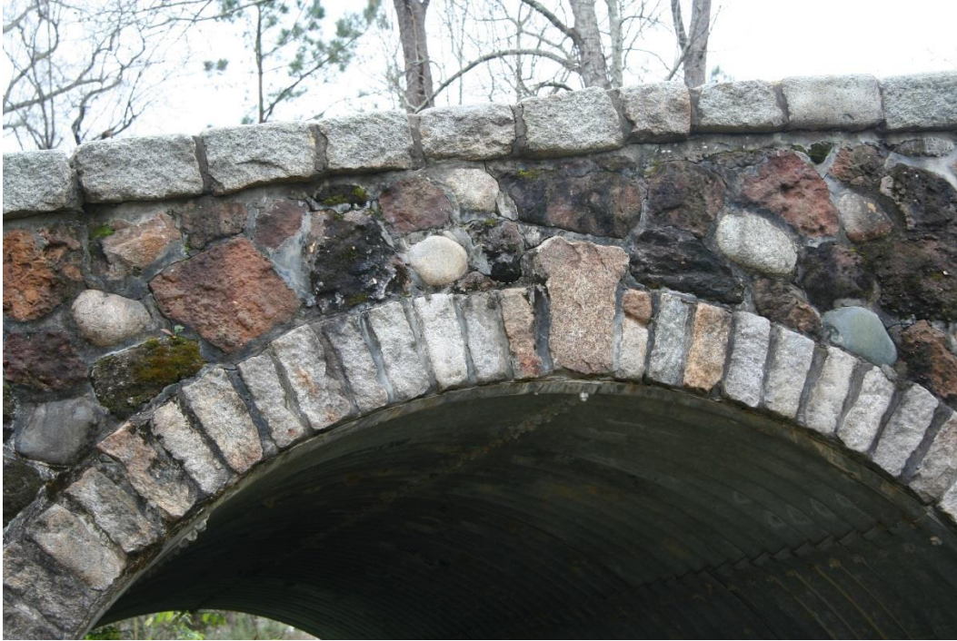
Condition Photo 7: Condition of mortar and stonework.
