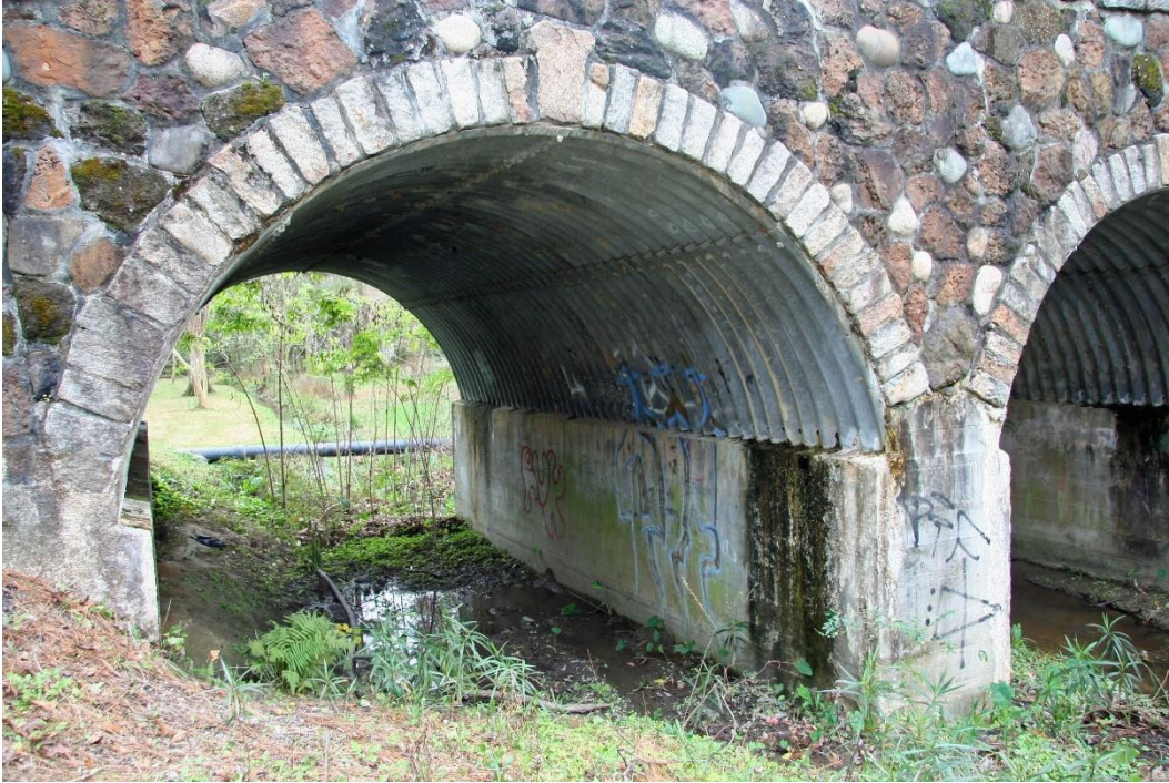
Character-defining Feature Photo 1: Design and construction of a galvanized, corrugated, metal, multi-plate arch culvert with arches consisting of multiple liner plates that comprise the arch barrels.
