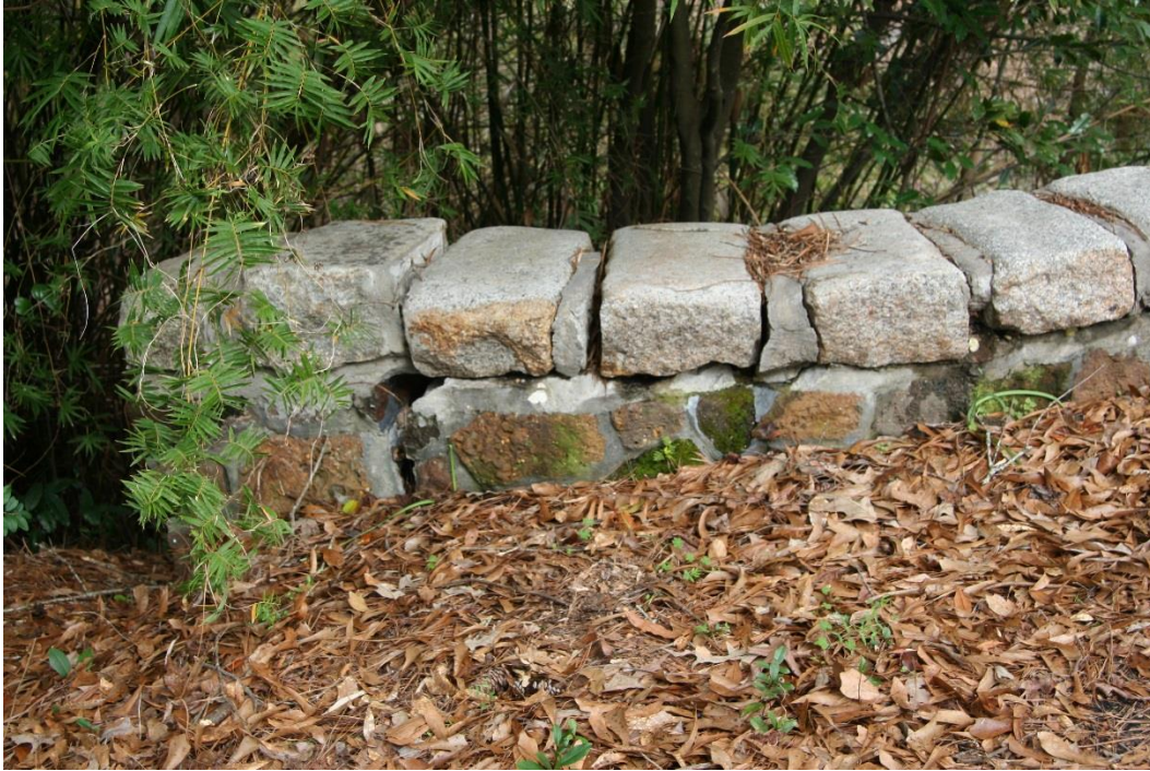
Condition Photo 13: Condition of mortar joints on northwest wingwall and capstones.
