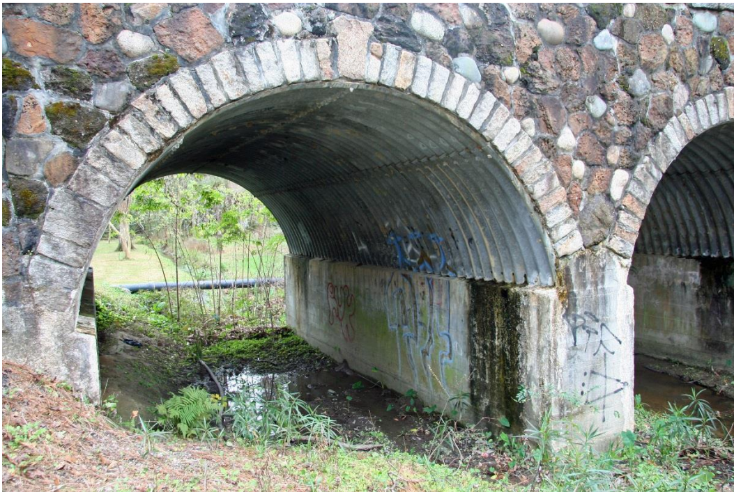
Condition Photo 8: Condition of easterly arch span; note graffiti on arch metal liner plates and cast-in-place concrete foundation walls.
