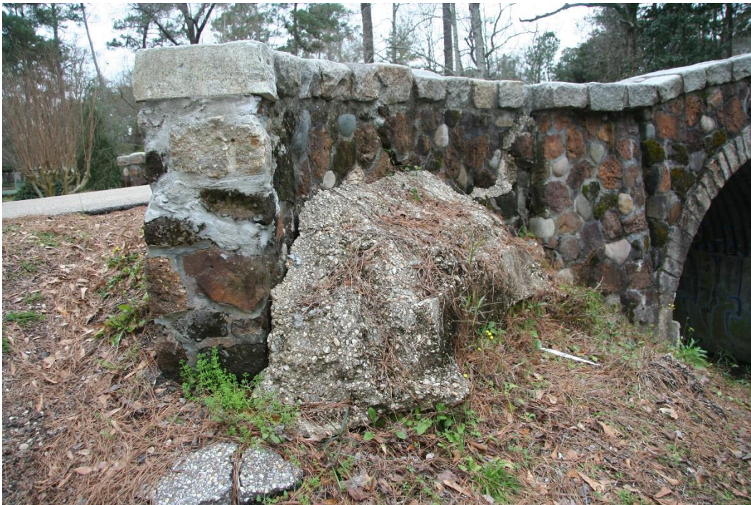
Condition Photo 6: Northeast wingwall; note mortar joints repairs and large chunk of concrete.
