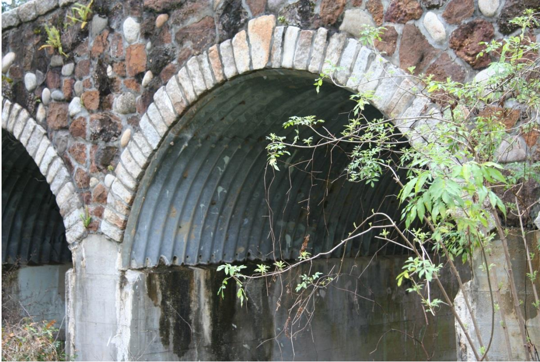
Condition Photo 5: Metal liner plate, stonework, and cast-in-place concrete foundation wall details.
