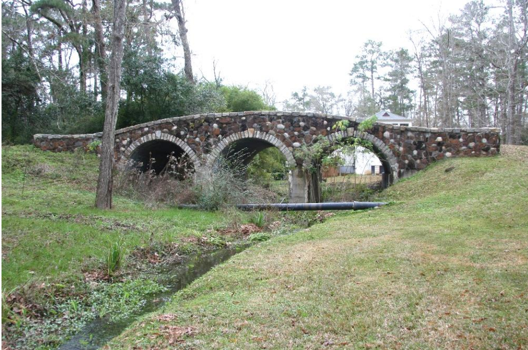
Condition Photo 1: Profile view of south (upstream) side of bridge, looking north.
