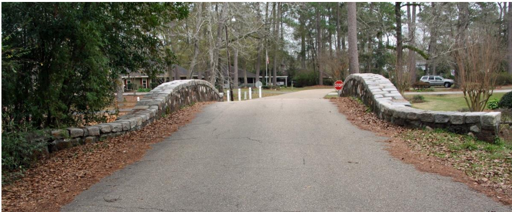
Condition Photo 10: Looking east across the bridge; note debris along parapet railings.
