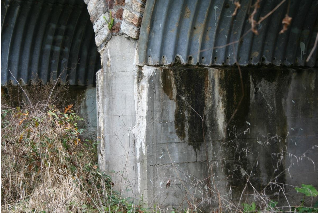
Condition Photo 11: Condition of cast-in-place concrete foundation walls and metal liner plate detail.
