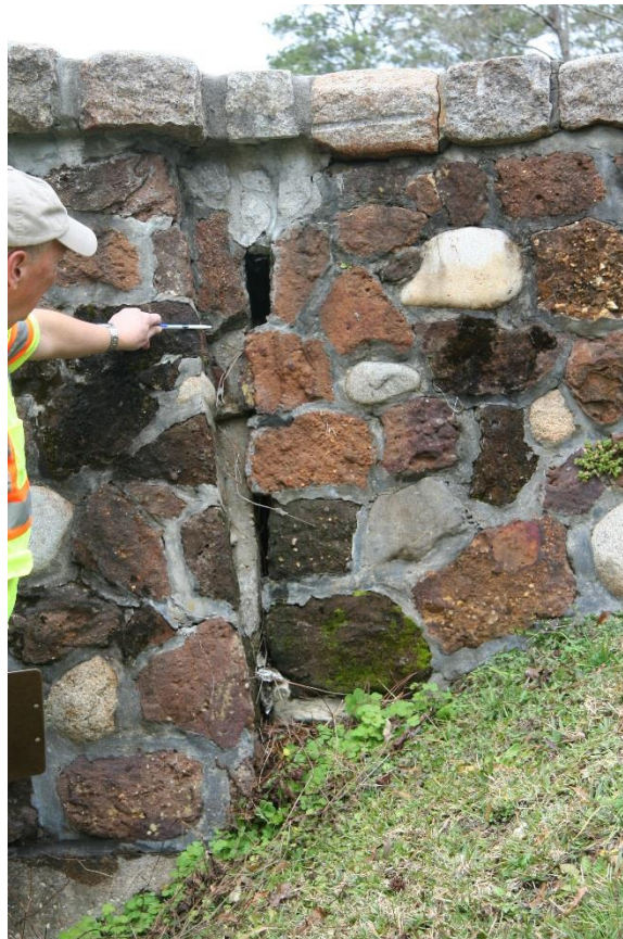
Condition Photo 12: Condition of southeast wingwall stones and mortar joints.
